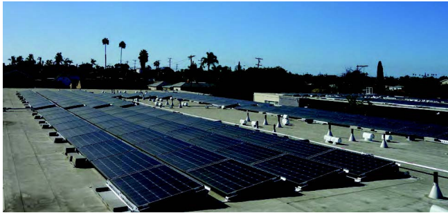
Figure 10. Rooftop Solar System on San Diego Supportive Housing Property
